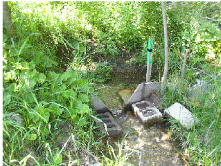
Figure 9 Drainage from the spring close to Well 5. Top: the creek on the south side of the road leading to Well 5. Bottom: the gauging structure at the point where the south creek spring emerges from the culvert and joins the north spring creek. This point is 60 m from Well 5.
