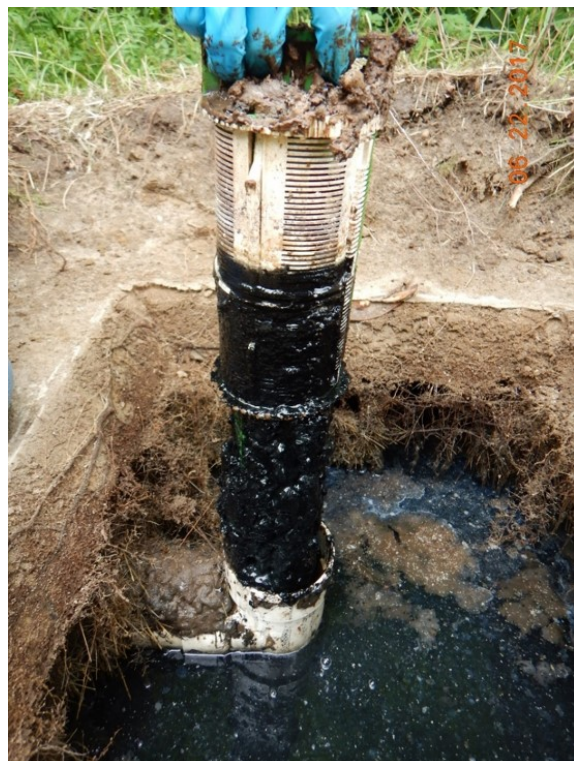
Figure 2. Dirty effluent filter requiring remedial action [Photo credit: Mississippi Rideau Septic System Office]
