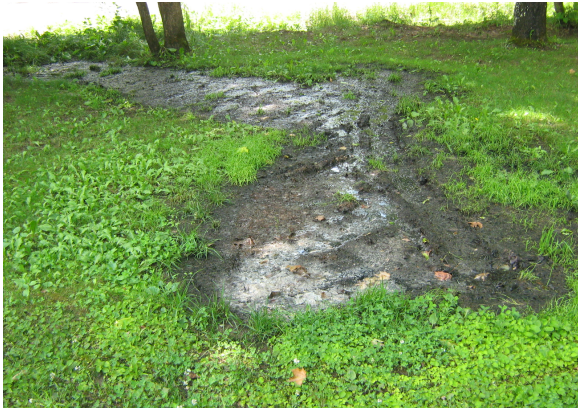
Figure 3. Example of a system that received a failed inspection [Photo credit: NBMCA]
